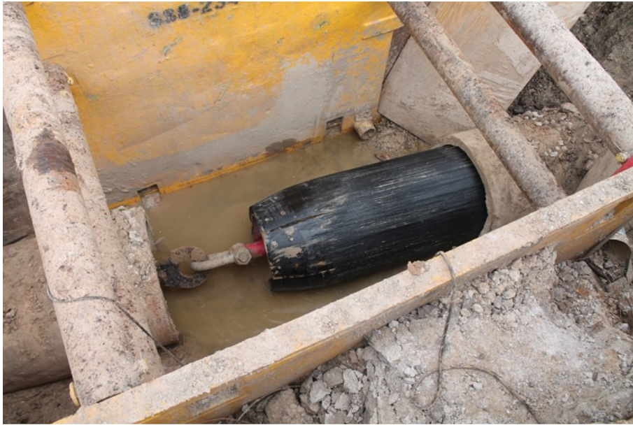
Trenchless refurbishment of old metal pipeline by “sliplining” with PE100. (Photo: PE100+ Association, PR004)
