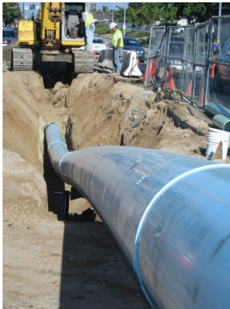
Trenchless refurbishment of old pipeline with welded PE100 pipes. (Photo: PE100+ Association, PR004)
